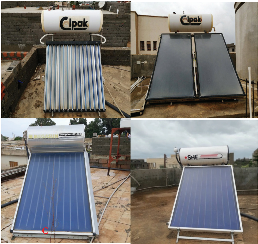
Figure 1 A sample of Investigated SWH systems installed in Tripoli-Libya. A: Calpak (FPC), B: Calpak (ETC), C: SHE (FPC) and D: Megason (FPC)
