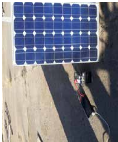
Figure (3). Solar PV cell for operating Air blower.
