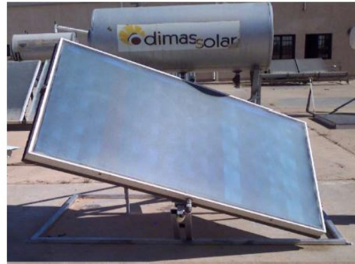
Figure (6). Overall tracker and thermosyphon system.
