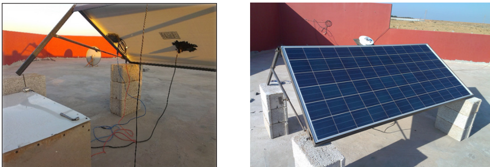
Figure (2). Photovoltaic modules mounted at an angle of 32.7° are situated on the top of a building in Derna, Libya
