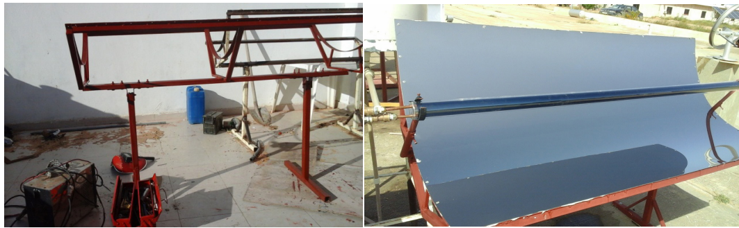
Figure (2). Metal structure of the parabolic trough collectors
