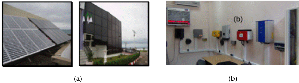
Figure 1 (a) Crystalline silicon PV panels (c-Si, m-Si) on rooftop and thin-film (a-Si, m-Si) on the facade of the UDES building. (b) The control room of the multi-technology PV power plant is connected to the UDES grid.
