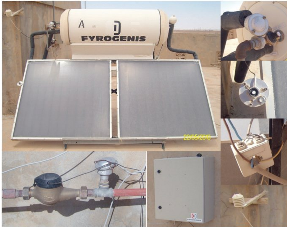
Figure (10). Solar water heater equipped with measuring sensors and data logger
