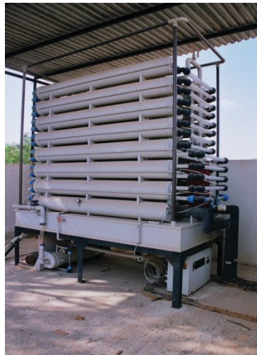
Figure (8). A view of the MSF desalination unit [4].
